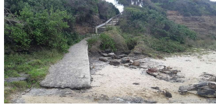
Berrara - Erosion due to runoff
